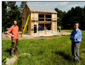
Gordon Chibroski/Staff Photographer Matthew O'Malia of G.O. Logic LLC stands in the natural field at the energy-efficient home being built in Belfast. The owner of the house — expected to cost about $225,000, excluding land — will not pay anything for heat or hot water, the developers say.
