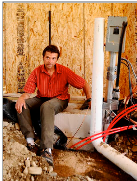
Gordon Chibroski/Staff Photographer Alan Gibson shows the single entry point for the utilities embedded in the insulated concrete floor of the Belfast home he's helping build.
