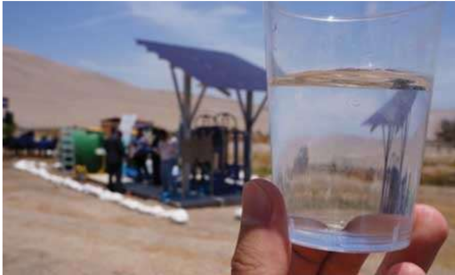
Transparent technology: the Lluta Valley project uses membrane separation technology to remove salt from the water, all powered by solar photovoltaic panels
