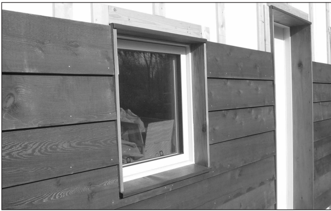
Figure 2. The exterior polystyrene partially laps the window frames. The builder used exterior jamb extensions and wood window sills to trim the edges of the polystyrene and the rainscreen strapping.
