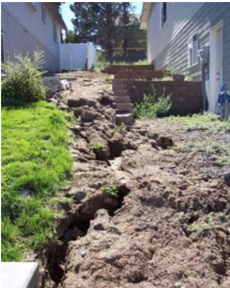
Erosion caused by stormwater
